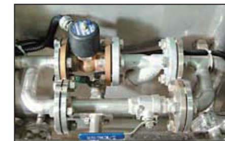
蒸汽控制閥 Steam Control Valve
