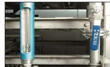
冰水流量計 Chilly Water Volume Meter
